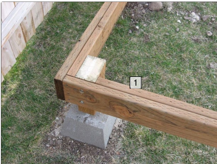
1. Placed internally, rather than externally along this wall.
